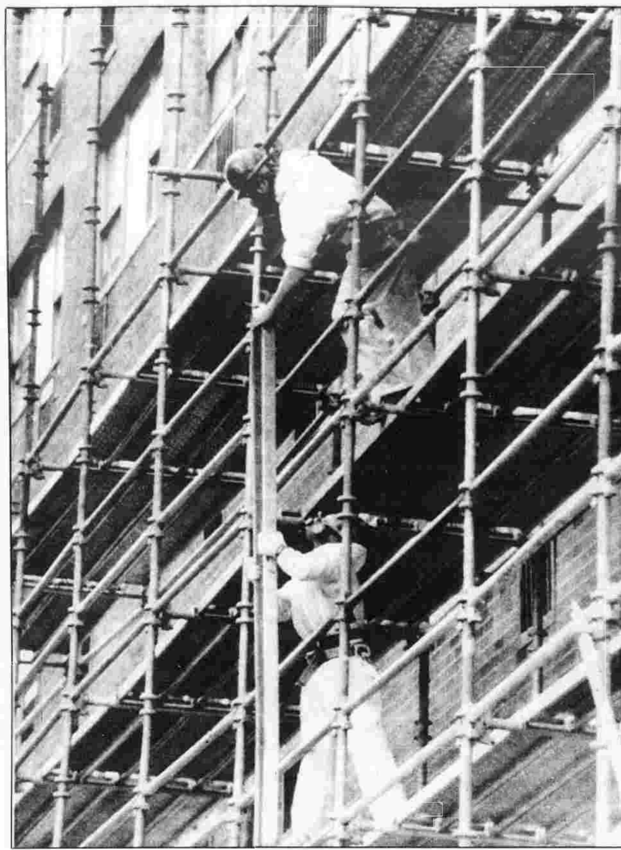
CLEANUP BEGINS - Workers wearing masks begin to construct what will be a plastic bubble around a 19-story apartment building in New York City Monday. The bubble will be used during removal of asbestos-laced mud left in the building after an explosion earlier this month of an underground power utility steam pipe, which sprayed steam, mud and debris.
